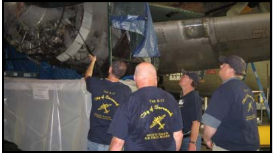
B-17 Volunteers testing the new steam cleaner after having received instructions from the company representative. Pictured: Glenn Braselton (operating spray nozzle), Jim Grismer, Bill Burkel, and JEB Harper
